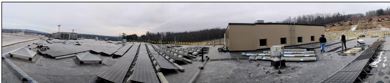
Solar PV system on the roof of the new Correctional Facility for Women in Concord, New Hampshire
