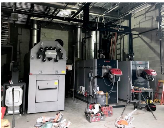
UNH Biomass Boilers & PDC Storage
